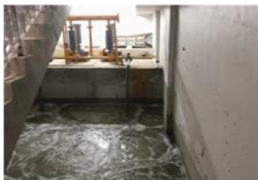
STP EXTENDED AERATION
