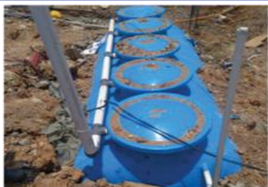
STP BIOFILTRATION FRP
